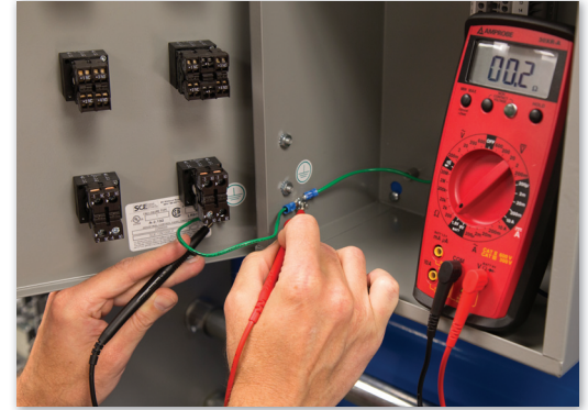
Voltage Check Using Multimeter
