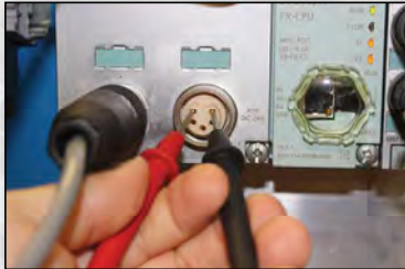
Supply Voltage Test
